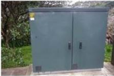
FTTN Cabinet - copper network
